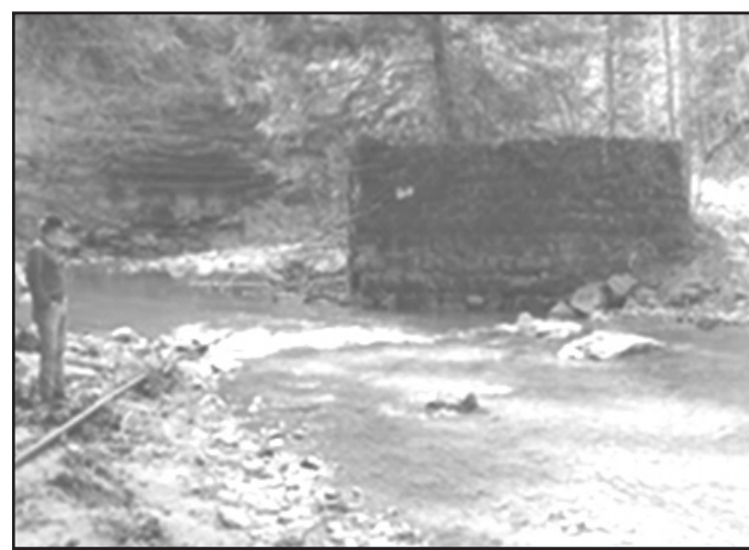
Remnants of a stone masonry bridge abutment on the former KN's line across Big Sinking Creek near Simcoe in Lee County. Note the old crude oil pipeline in lower left of the picture.
