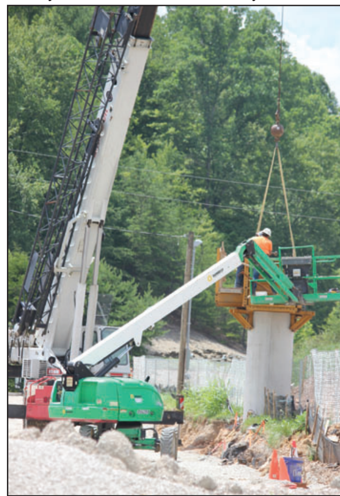
Construction workers for the new Area Technical Center have been constructing pillars for the pedway that will connect the ATC to the high school.
