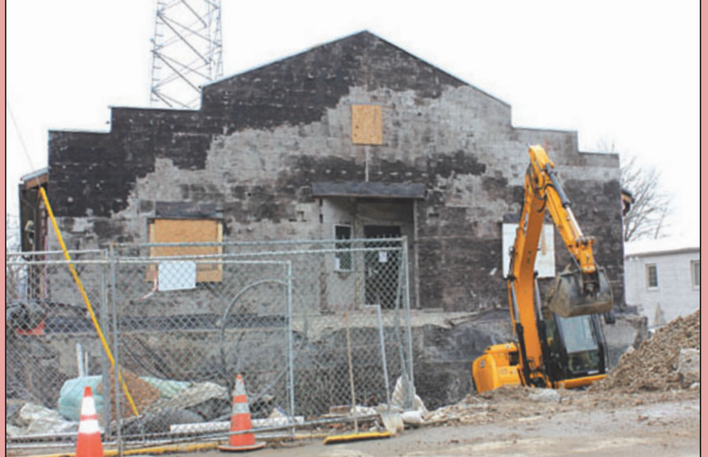
Contractors worked Monday on building a safe room onto the Emergency Operations Center on Broadway. When completed, the room is expected to withstand winds of up to 250 miles per hour. During tornadoes, dispatchers and emergency personnel will be able to keep working while inside the room. The safe room construction bid was awarded to Riddell Construction of Irvine, the original contractor of the EOC Center. The safe room construction is funded with CSEPP funds.
