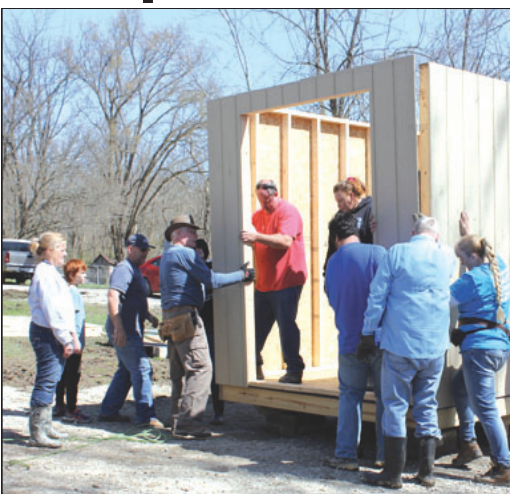
Volunteers put up the last wall on a storage building in Ravenna. This wall was the one with the opening for double doors. The walls were already built when they arrived in Irvine last week. All other parts were pre-cut to make assembly in a day easier.
