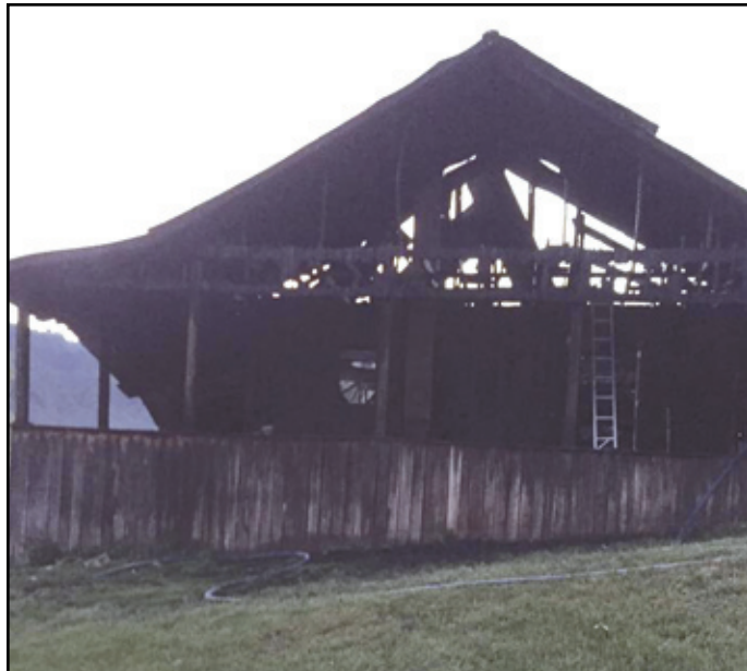
The above photo shows all that remains of the Neal home on Campbell's Branch after a house-fire on Saturday.
