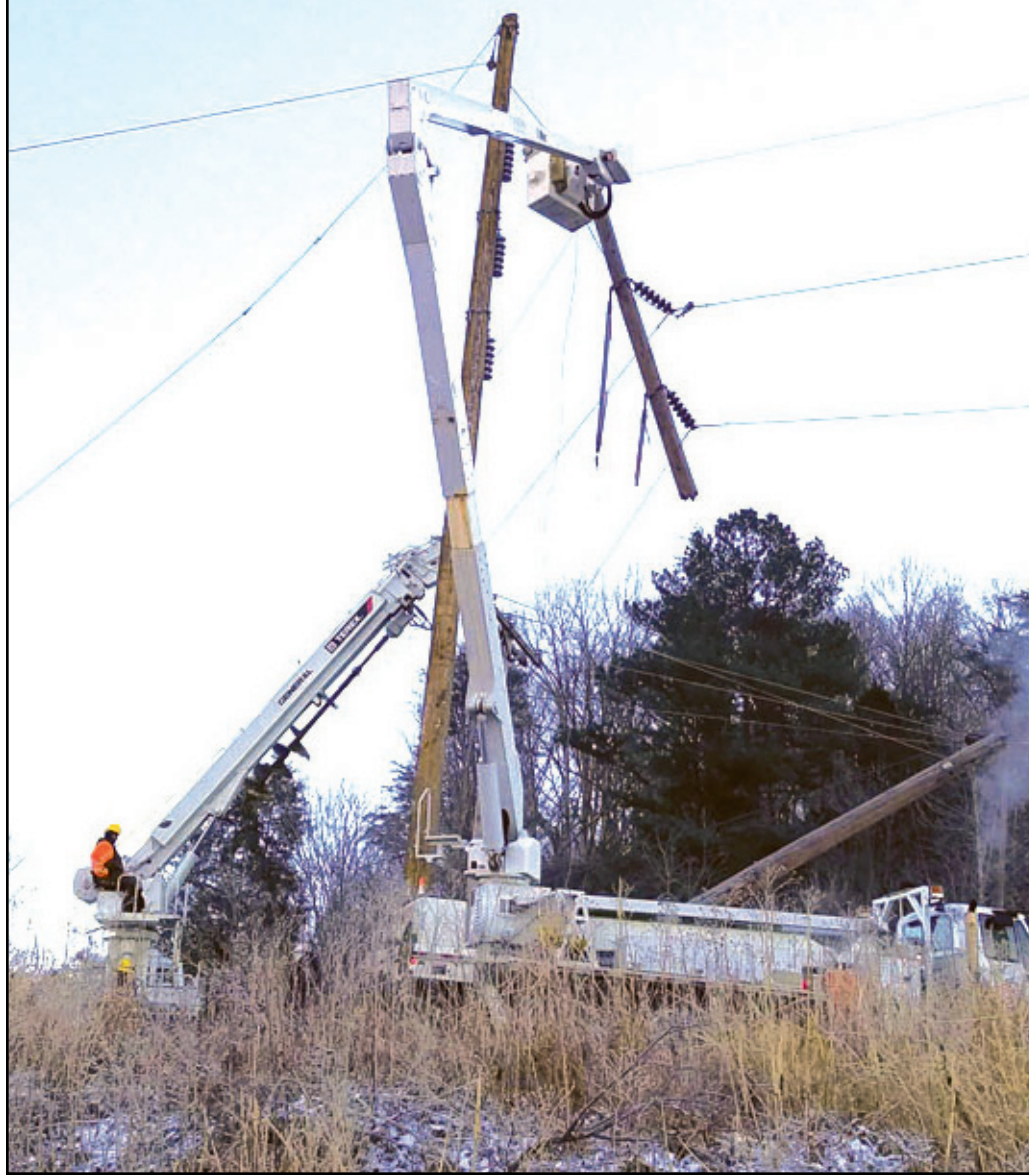
KENTUCKY UTILITIES contractors replace a broken transmission pole off KY HWY 52 near Irvine. A vehicle hit the pole and resulted in an outage that impacted families in Estill, Lee, Powell and Wolfe counties. Photo by Brent Arvin
