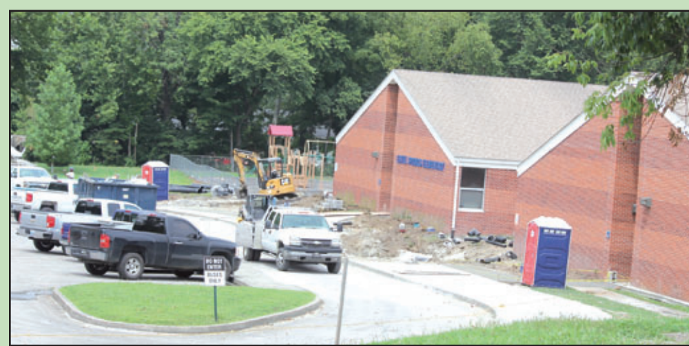
The first day of Estill County Schools for students has been rescheduled for August 13 due to construction at Estill Springs Elementary. The photo was taken Monday of the main entrance to the school.
