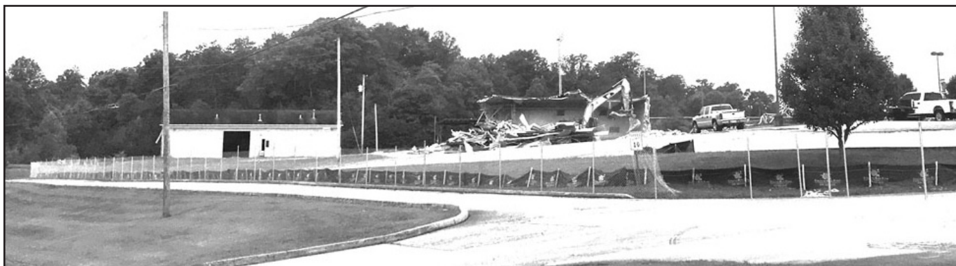
Demolition of the old Estill County Schools' garage was nearly complete on Tuesday. (Vicki Horn photo)
